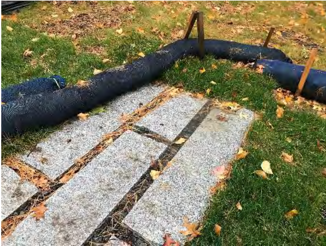
Fig 1: The level spreader below the manhole at Gundalow Landing/east side of the bay. Viewing southwest. (10-13-20)
