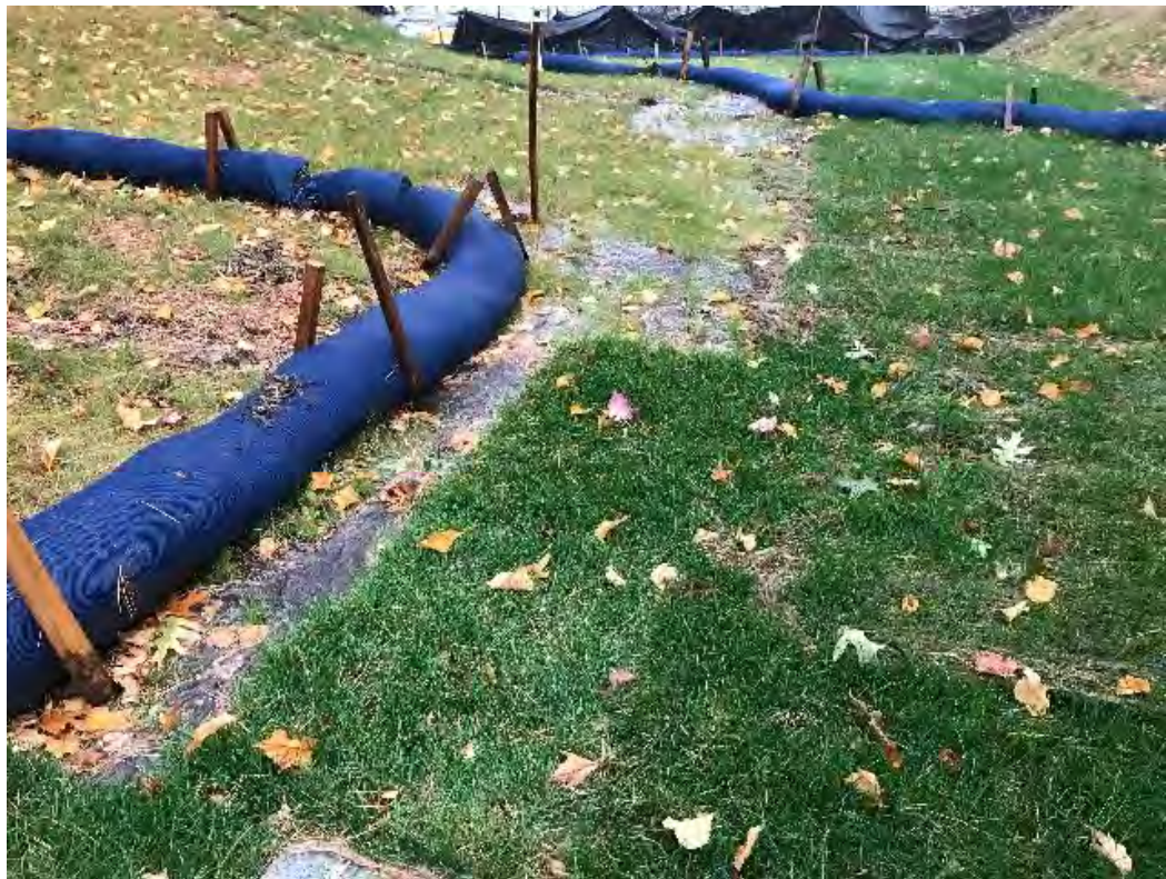
Fig 2: Initial positioning of silt sock along the southeastern side of the slope below the manhole at Gundalow Landing. Viewing southwest. (10-13-20)
