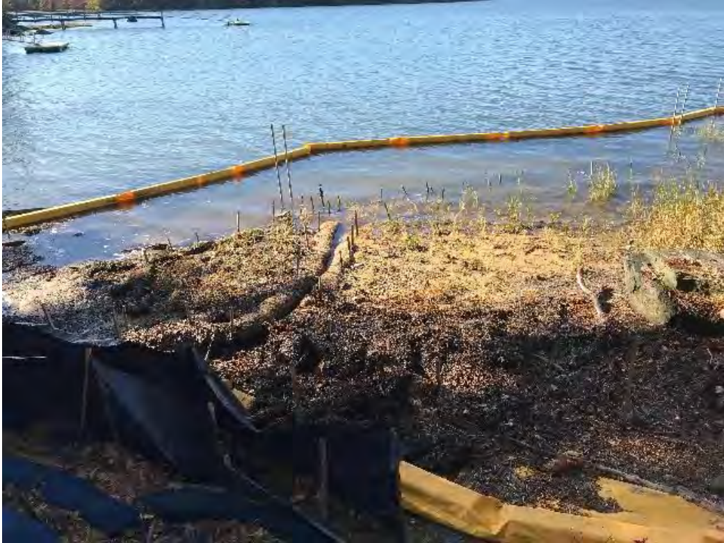
Fig 9: Salt marsh restoration at Gundalow Landing/east side of the bay. Viewing southwest. (10-14-20)
