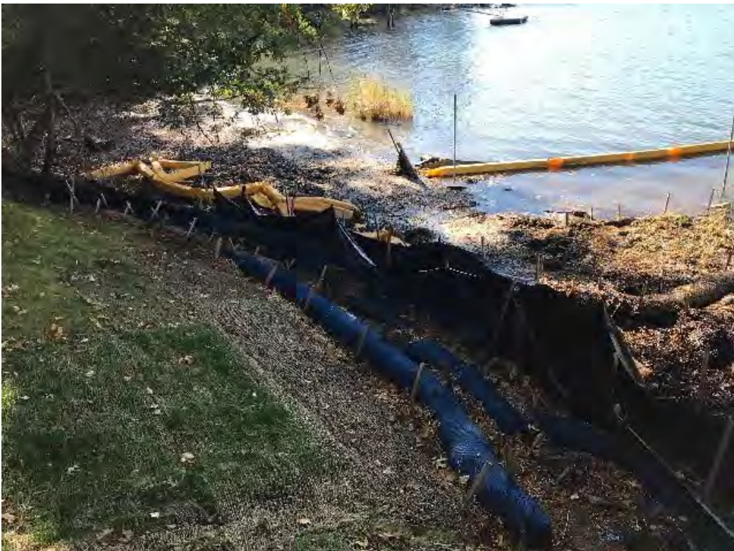
Fig 8: Toe of the slope below the manhole at Gundalow Landing/east side of the bay. Viewing south. (10-14-20)
