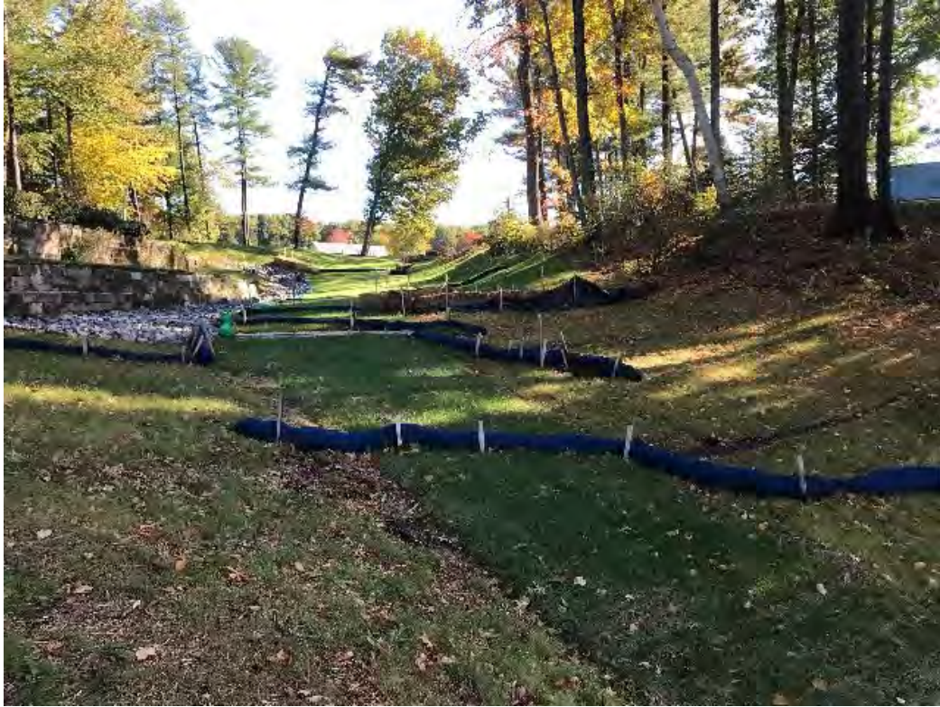
Fig 7: Slope below the manhole at Gundalow Landing/east side of the bay. Viewing east. (10-14-20)
