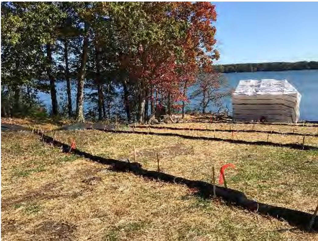
Fig 10: The slope above the cable house at the Eversource property/west side of the bay. Viewing east. (10-14-20)
