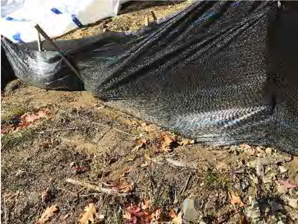
Fig 13: Silt fence needing repair along the toe of the slope north of the cable house. Viewing southwest. (10-14-20)
