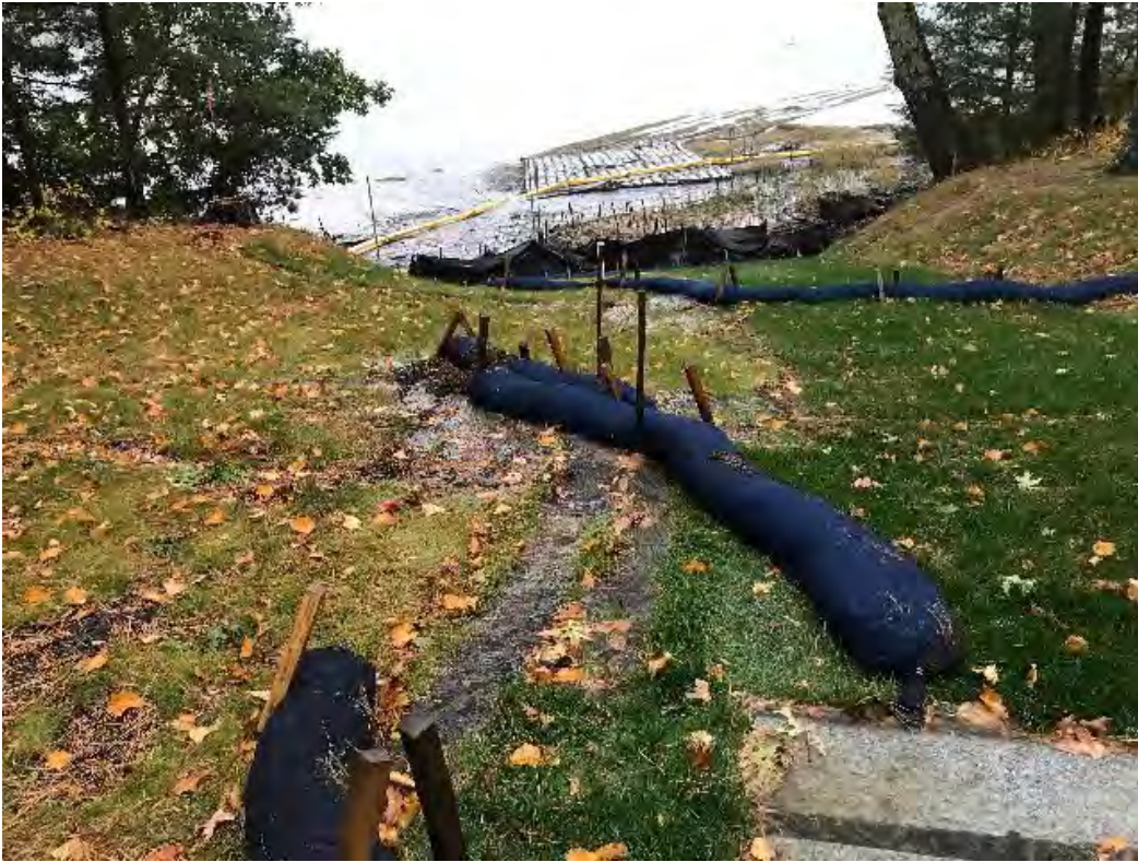
Fig 3: Adjusted positioning of silt sock along the southeastern side of the slope below the manhole at Gundalow Landing. Viewing southwest. (10-13-20)
